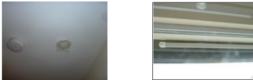
Figure 4: All trickle air vents, mechanical air vents, and kitchen hoods were sealed off; mechanical ventilation air ingress and egress points were also sealed and the systems switched off before air pressure and air leakage tests.
