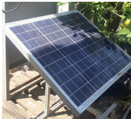
Gambar 3. 6 Polycrystalline silicon solar cell
